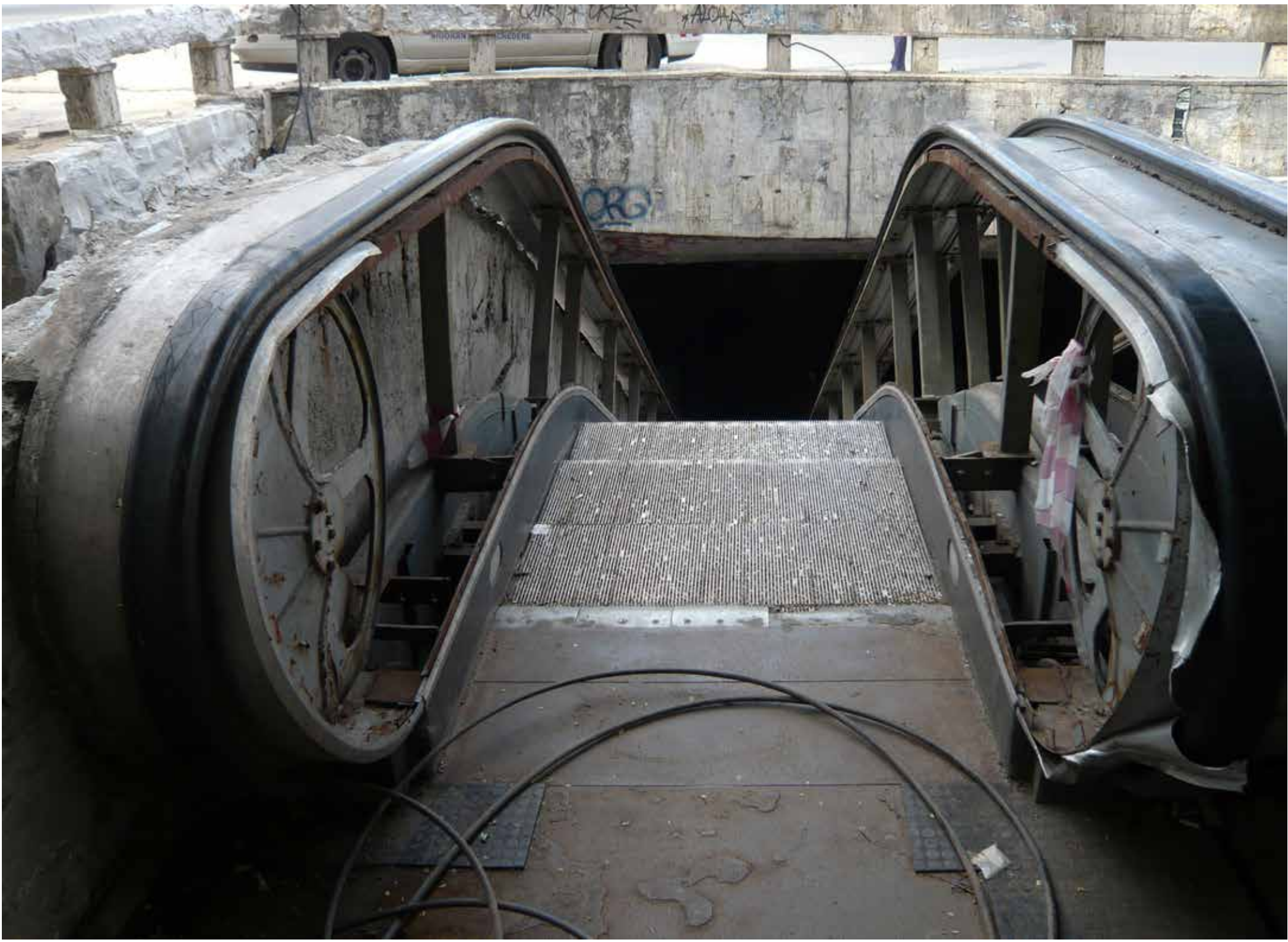
off the road – escalator
